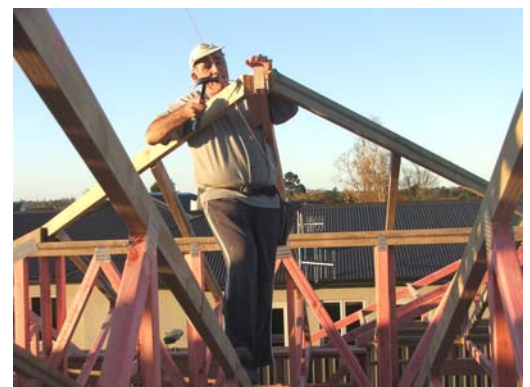
Bill Todd 'on the job' building Donald Stevenson's new house in Hastings
